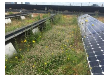
The green roof 4 weeks after being irrigated and covered in Haresfoot clover, hawks beard and cats ear flowers.
